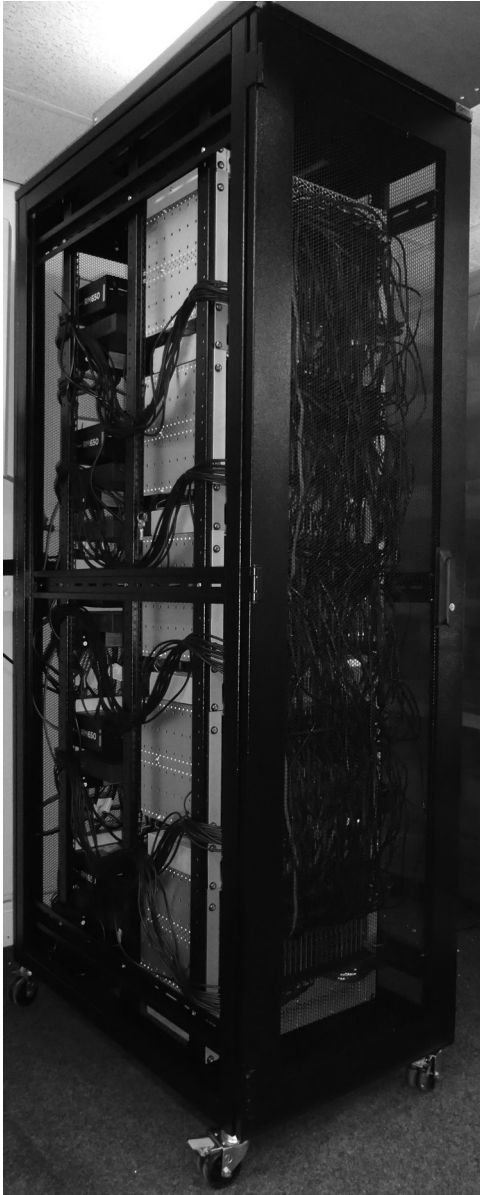
Fig. 2 SpiNNaker cabinet incorporating over 100,000 ARM processor cores
